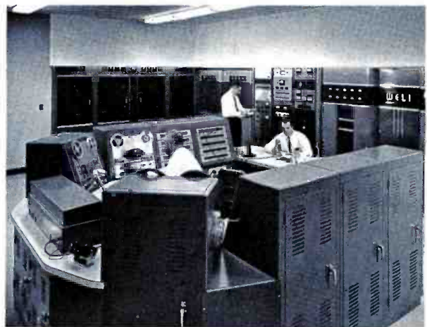
The finest control equipment
